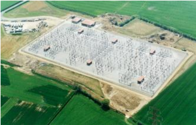
AIS (Air Insulated Switchgear)
