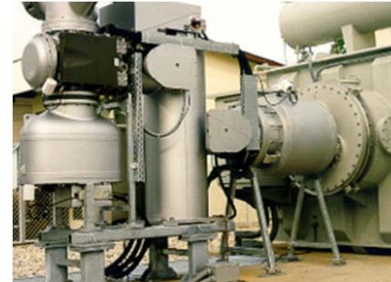
Transformer direct connection
